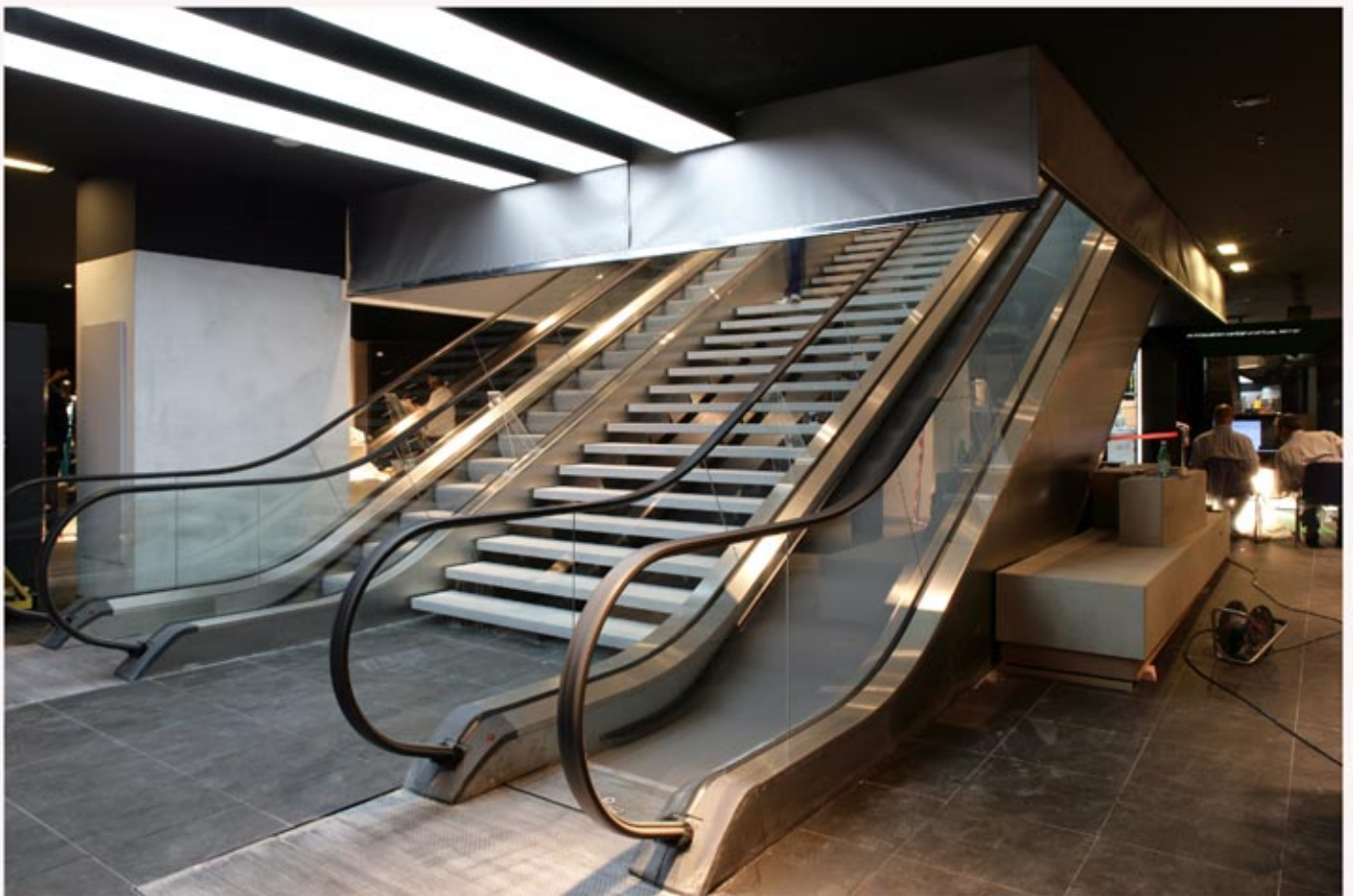
Coopers smoke curtains protect the central escalators in the new Adidas Sport Performance store in Paris
